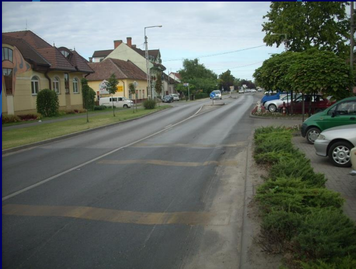
Pavement condition - rutting
