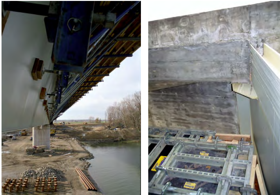
Figure 4.62 Outer support of the concrete slab and the connection of the concrete slab and steel girder.
