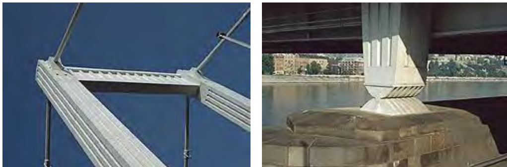
Figure 4.26 The new pylon, similarly to that of the old structure, is hinged. The original hinges were re-used.
