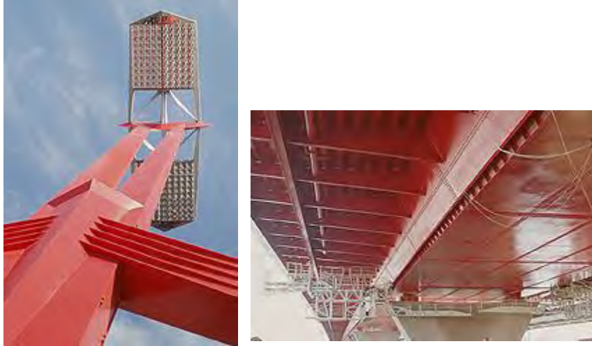
Figure 4.51 One of the lightening pylons with the mirrors and the erection of the lightening system.
