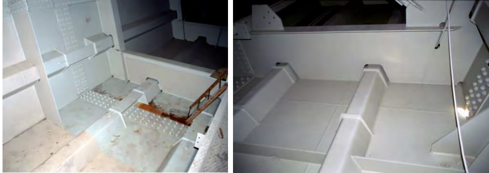
Figure 4.61 In-situ connection of steel bridge and lower flange plate of composite bridge.
